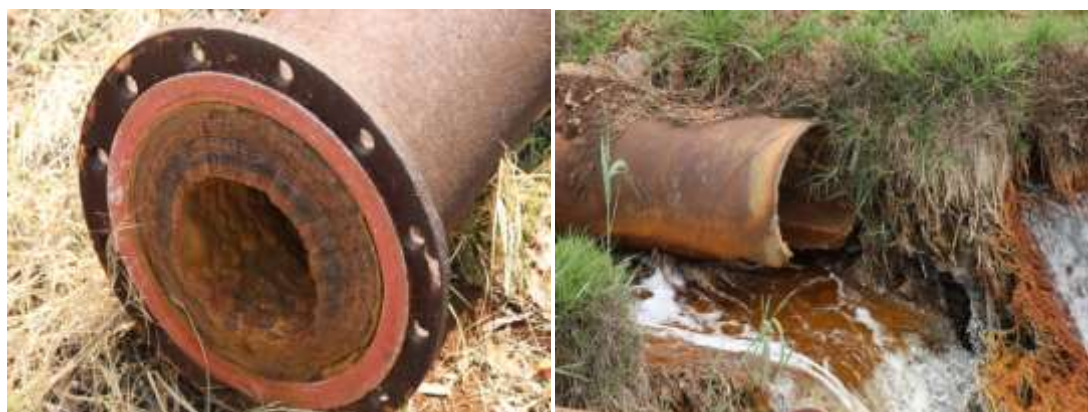
Pipes transporting Acid Mine Drainage . The photograph on the left shows a pipe with precipitated metals and the photograph on the right shows corrosion caused by Acid Mine Drainage .
